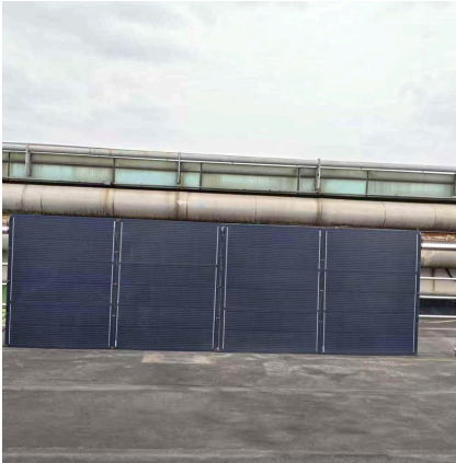
800 W balcony system
